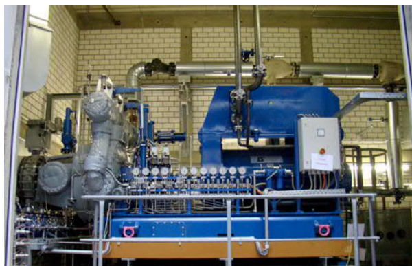
Figure 3.6 – Steam turbine (source: Spilling Technologies GmbH)
