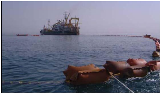
Figure 15: Cable with cable floats
